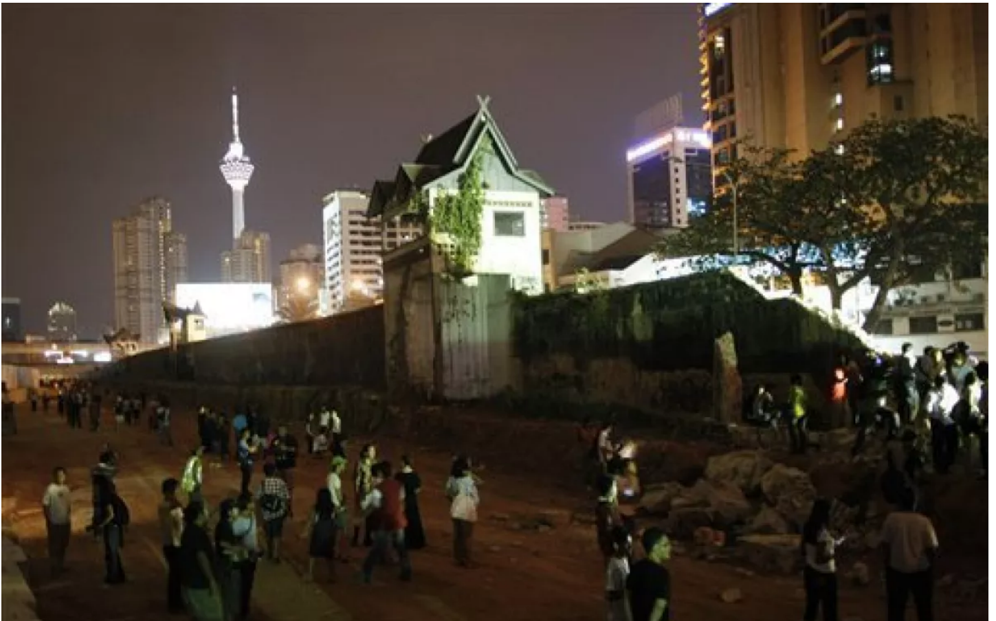
The 394-meter-long wall of Pudu Prison which is being demolished in downtown Kuala Lumpur, on Monday June 21, 2010. A controversial plan to tear down part of a 115-year-old jail for commercial development in the Malaysian capital
